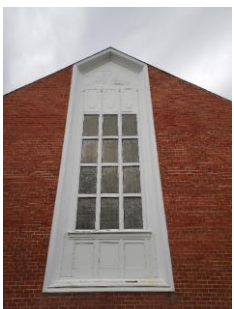
Before (damaged plexiglass)
